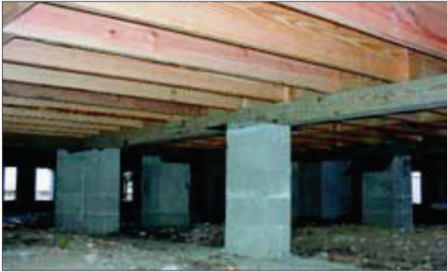
Treated Southern Pine 4x6 sill beams are supported by concrete block piers on a continuous spread footing.
