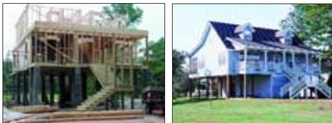
Storm surge protection in hurricane-prone coastal areas requires an elevated floor system. Wood piles are also an option for this application.
