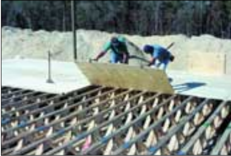
Workers install subfloor sheathing over floor trusses of a 5,000 sq. ft. assembly building. See case study D, page 43.
