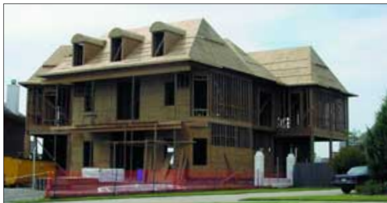
Optimum protection against Formosan termites is attained by using all pressure-treated Southern Pine kiln-dried after treatment (KDAT) lumber and sheathing for this 14,000 square-foot lakefront home in suburban New Orleans.
